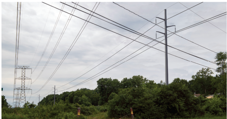
Photo simulation of the upgraded 115 kV line in New Windsor. Note that the other, larger 345 kV structure is not part of RTS and will remain as it is today.
